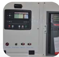
Control Panel & MCB
